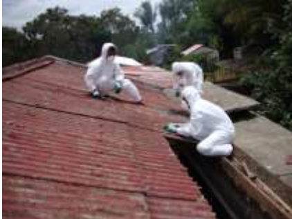
FLD staff working together to remove the asbestos roof on the Doctors house
